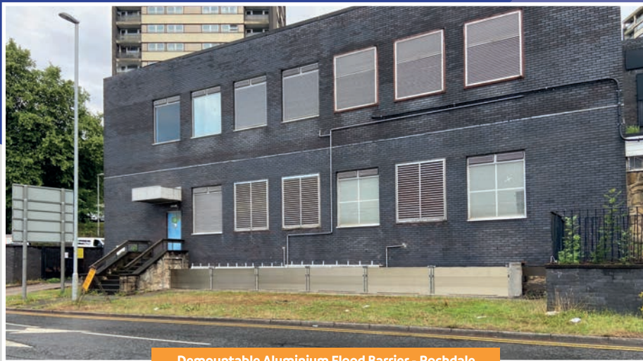
Demountable Aluminium Flood Barrier - Rochdale
