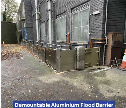
Demountable Aluminium Flood Barrier & Stainless Steel Flood Gate (Rear)
