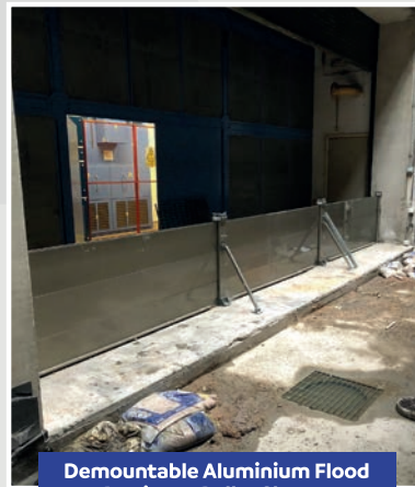
Demountable Aluminium Flood Barrier to Roller Shutter
