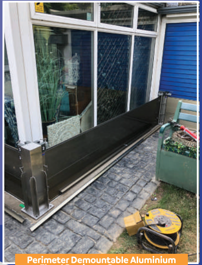
Perimeter Demountable Aluminium Flood Barrier to Conservatory
