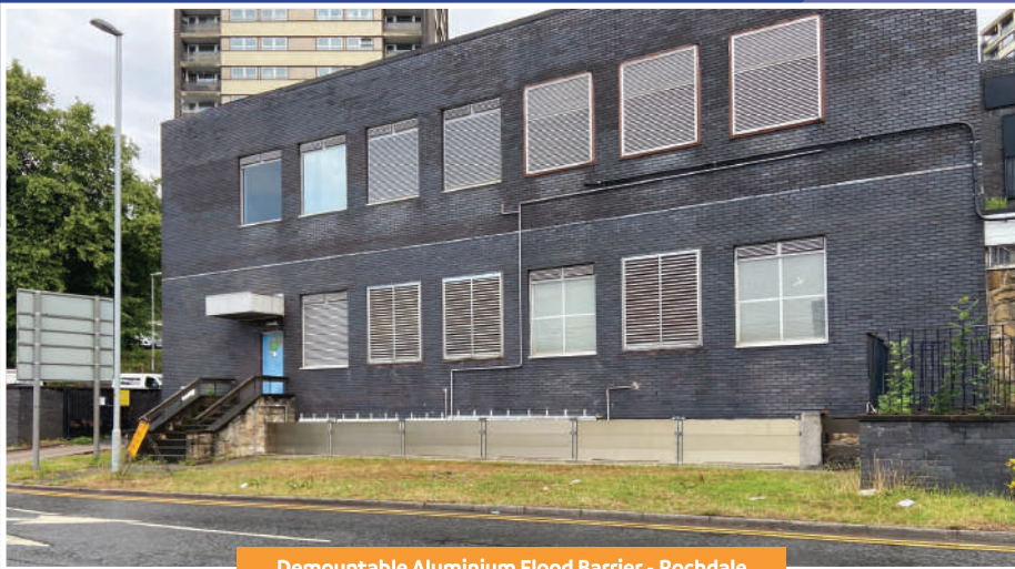
Demountable Aluminium Flood Barrier - Rochdale
